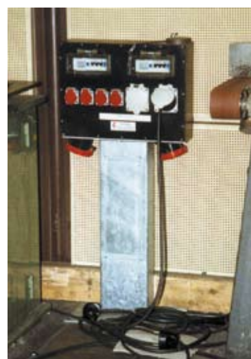
Power distribution for metalworking
