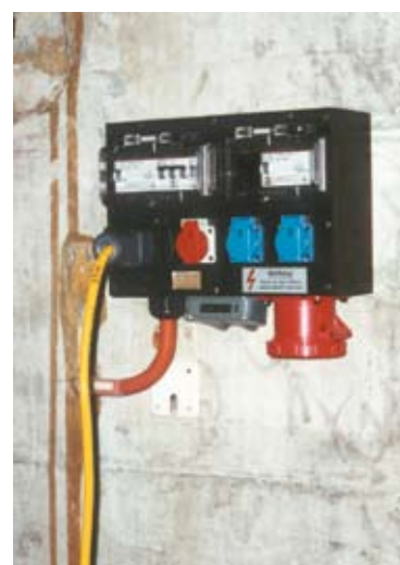
Power connections in factory yard
