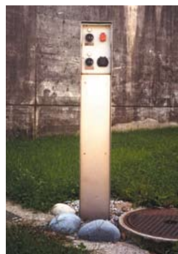
Control and power in V2A column
