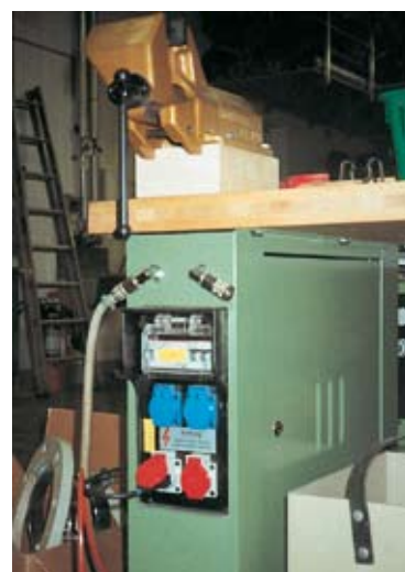
Power from workbench
