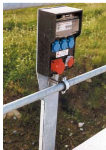
Electrical distribution with fixing, modified for the conditions
