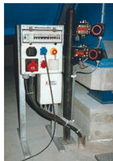
Power distribution for heating
