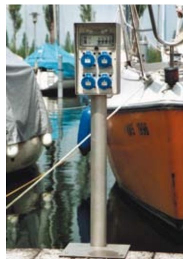
Power distribution on landing stages
