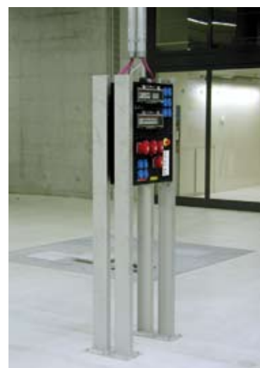
Power distribution 380/500 V for industry
