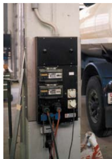
Power distribution in HGV shed
