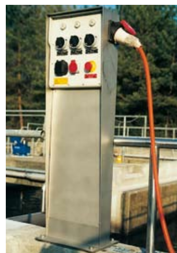
Control and servicing connections in V2A column
