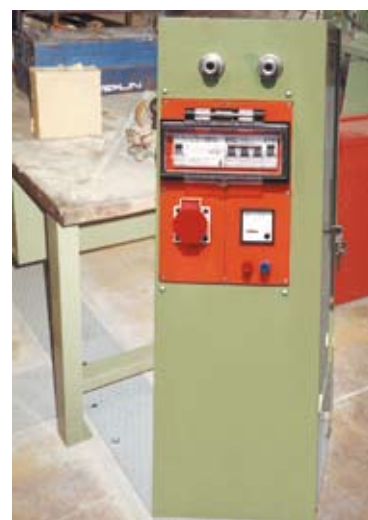
Workshop power distribution for testing
